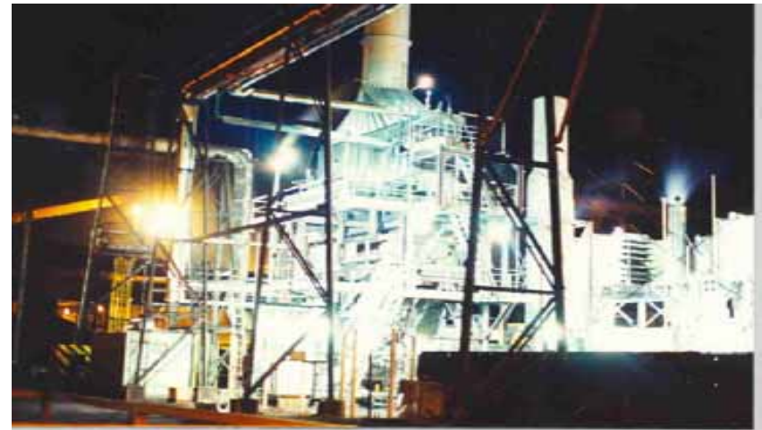
Designed, Manufactured, Installed and Commissioned By Senior
